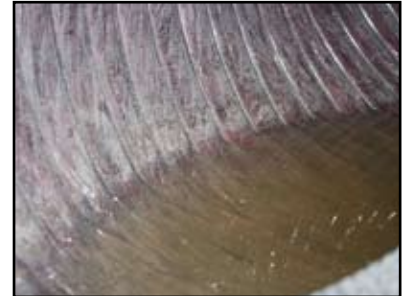
Accumulated condensation in typical 6" insulated flex duct
